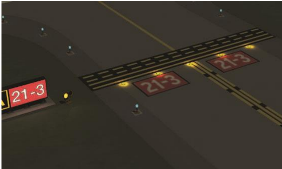
Figure 2-14: Runway Guard Lights (elevated and inset)
