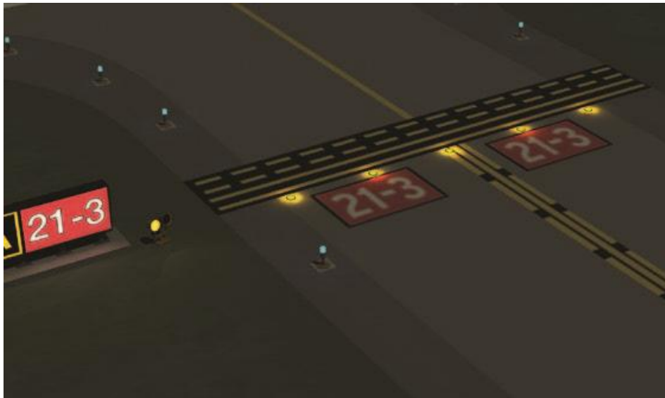
Figure 2-14: Runway Guard Lights (elevated and inset)
