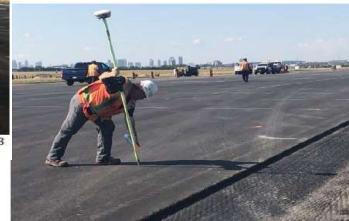
Stage 1C: Surveyor marking vertices of concrete slabs below asphalt for routing and sealing.
