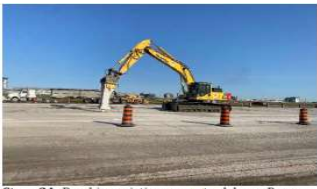
Stage 2A: Breaking existing concrete slabs on Runway keel section at Taxiway D5 intersection for removal.
