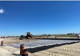
Stage 2C: Placement of granular base and installation of geotextile and geogrid.
