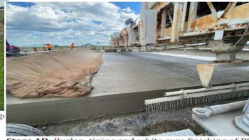
Stage 1D: Burlap, tining and white cure finishing of PCC slip form paving.
